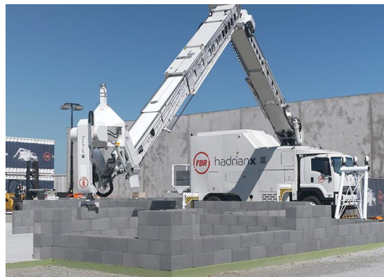
Figure 4. The Hadrian x uses linear mostly its linear actuators on a rotating platform to place bricks. (FBR construction, 2019)
