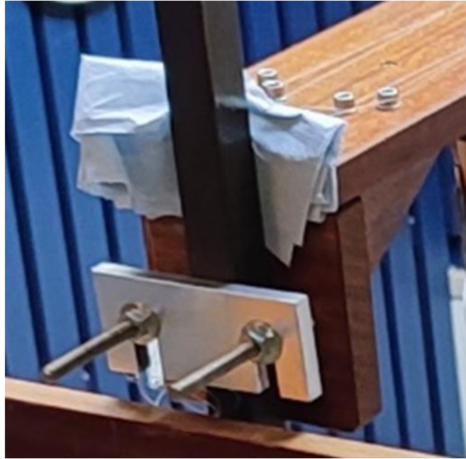
Figure 11: The metal fixing plank and the paper used to correct for the handrail inclination.
