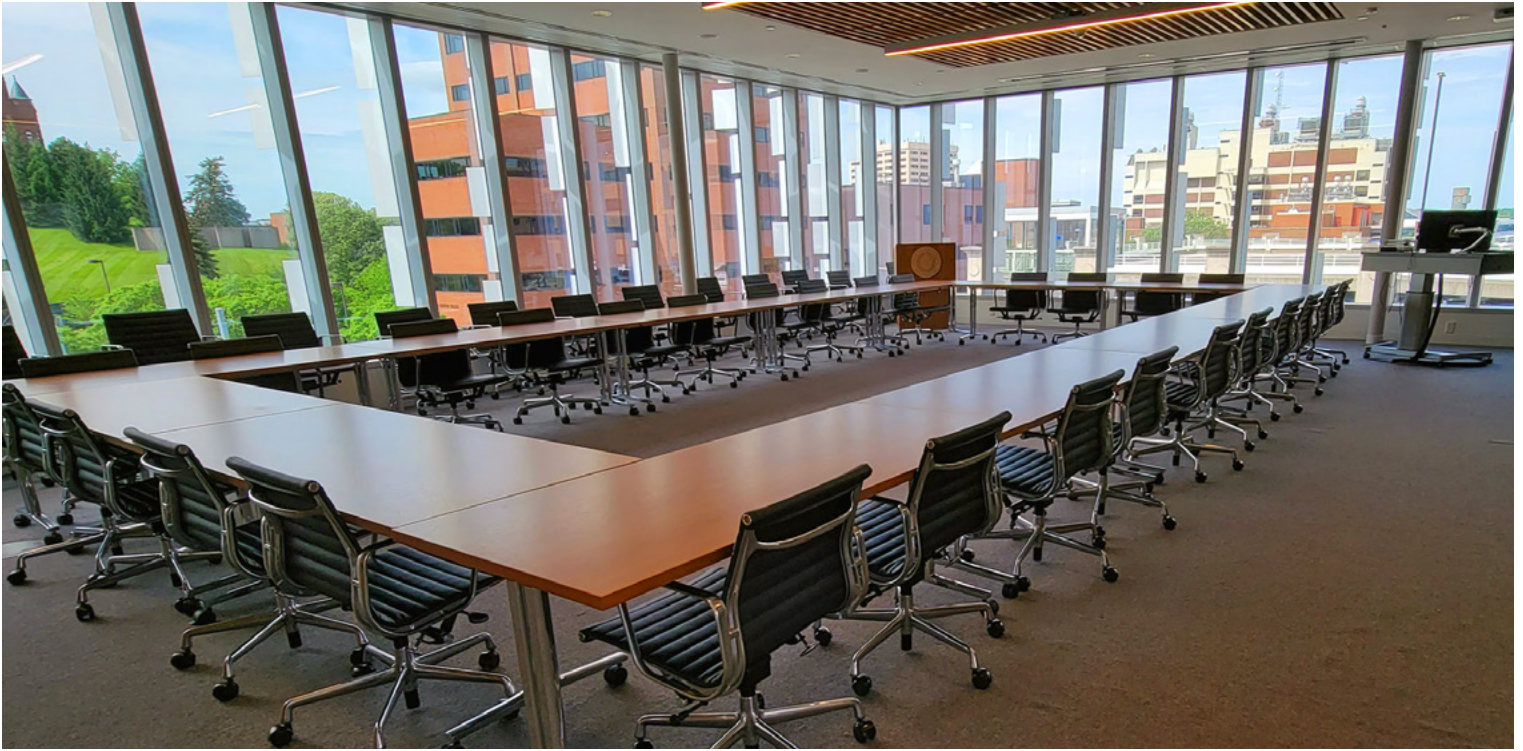
Meeting spaces such as Conference Room 330 include a DTP CrossPoint 4K scaling presentation switcher for signal routing, audio, and control, with the specific model dependent on room size and resources. All photos courtesy of Syracuse University, Steve Sartori.
