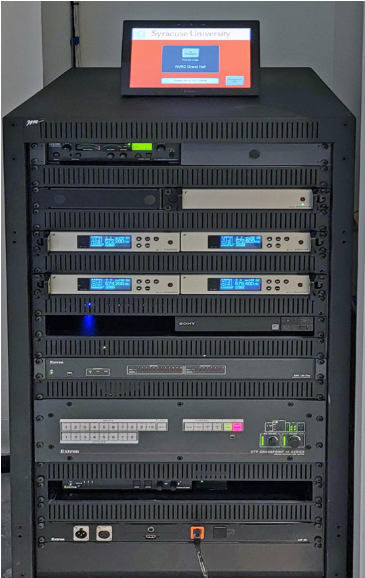
In the Grand Hall, the AV products are rack-mounted in an equipment room. An Extron TLP Pro 1025T 10" TouchLink Pro Touchpanel on the rack offers local system control.
