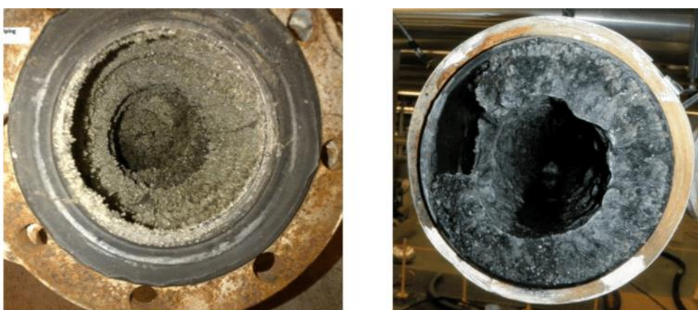
Figure 3. Formation of Struvite in WWTP pipes
