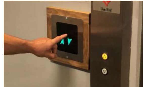
Schindler Elevator, U.S. Airport
