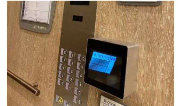
Mitsubishi Elevator, Hospital in Turkey
