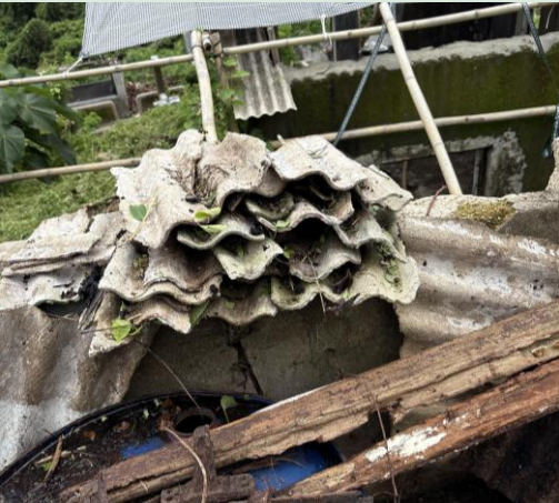
Corrugated roofing identified as asbestos-containing material
