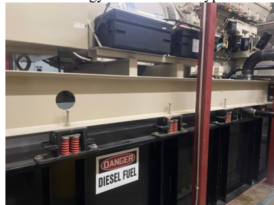
Figure 3: ThinkOn Data Centre's Diesel Generator, Photo by Lila Sparks
